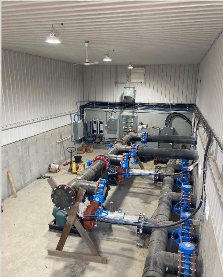
Station de pompage
