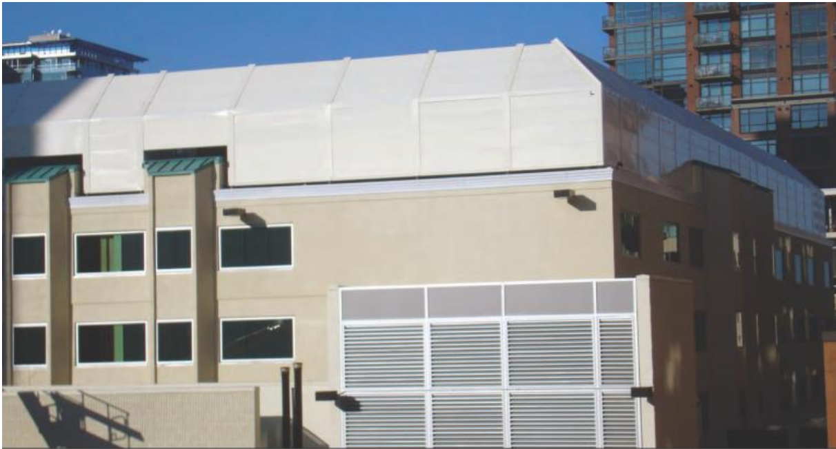
NOISEBLOCK™ wall system, Hospital Rooftop Equipment Yard
