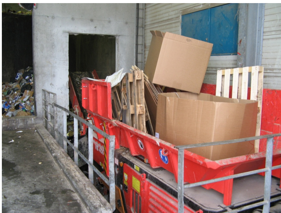
Picture 6 - Shredder on the Aasiaat plant
