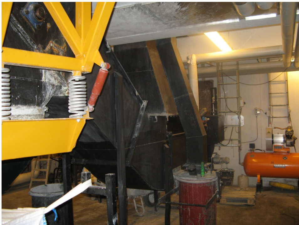
Picture 3 - Wet bottom ash scraper, vibrating conveyor as well as a bucket for grate riddlings
