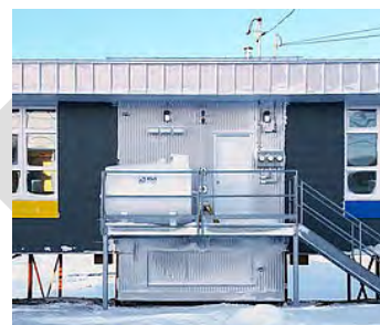
Figure 8: Furnace-oil heating equipment Source: SHQ
