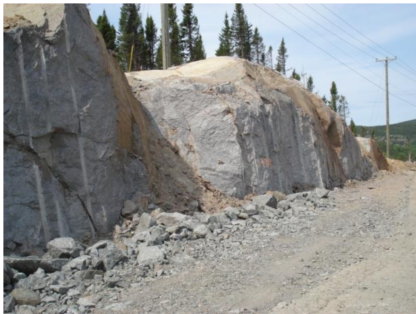
Figure 9-3: Wedge failure within pre-shear blasted rock face.
