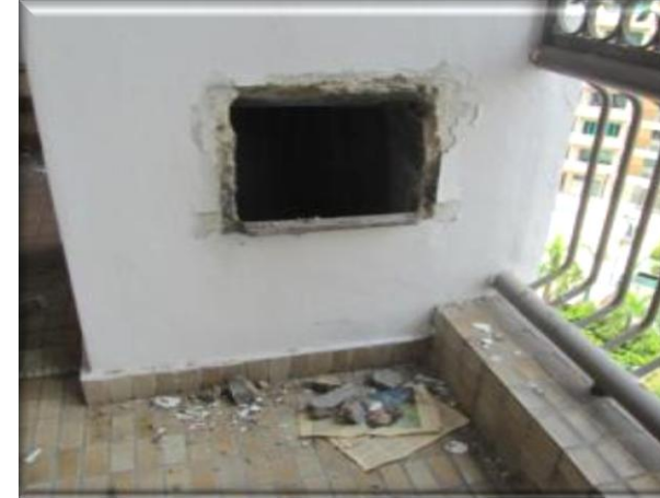
Rubbish chute insulation lining
