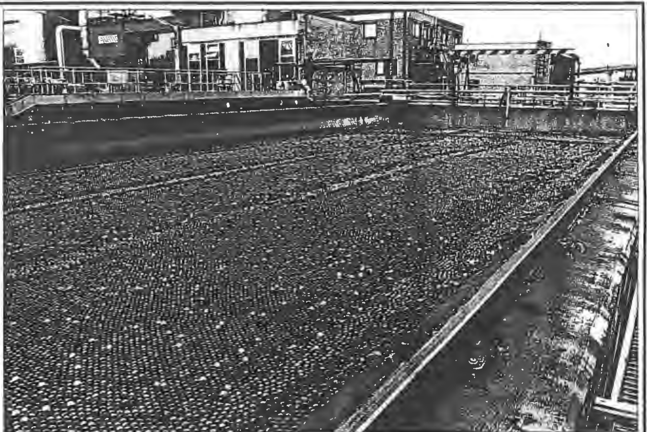
■ A sewage plant covered with an Allplas Ball Blanket (Diameter of balls is 45mm)
